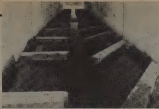
Concrete rectangular culvert with offset baffles bolted to the floor. The baffles were made of treated timber. Without them water velocities would be too high and the depth too shallow during fish migration.
